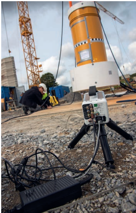
Set-up of the measurement instrumentation.
