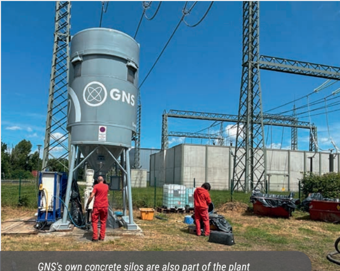
GNS's own concrete silos are also part of the plant technology for backfilling Konrad containers.
