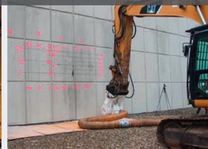
Detailed view of the milling head, excavator with mounted milling head in front of the test area for milling trials.
